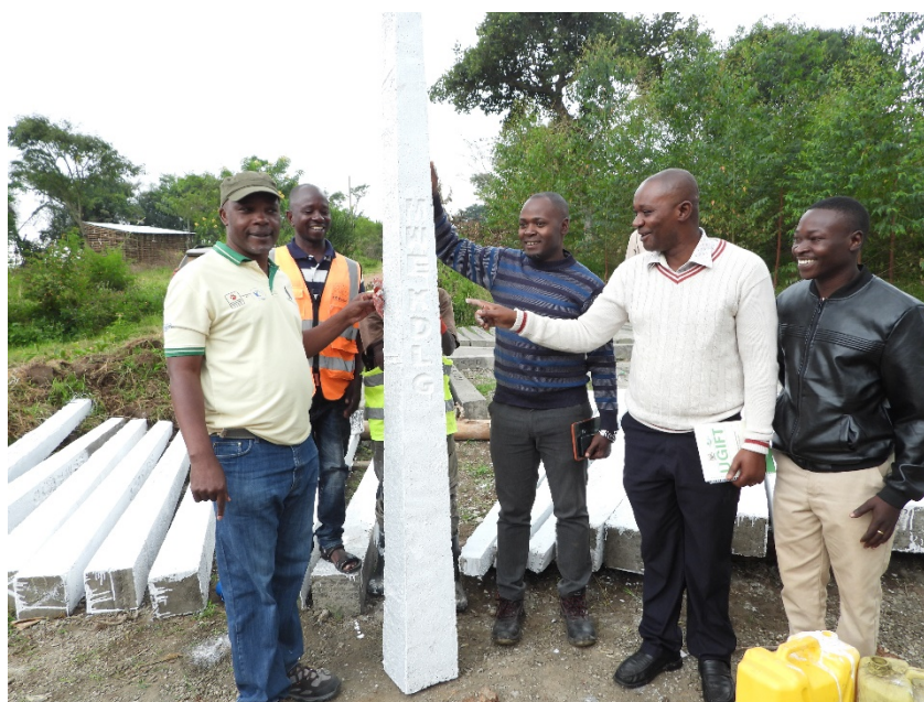
Figure 18: The Executive Directors of UBF and NU together with the District Environment Officer, Kamwenge District inspecting the concrete pillars made by Gampe Associate Engineering & Services Ltd for demarcation of boundaries of Rushango and Kajororo wetlands, Kamwenge district
